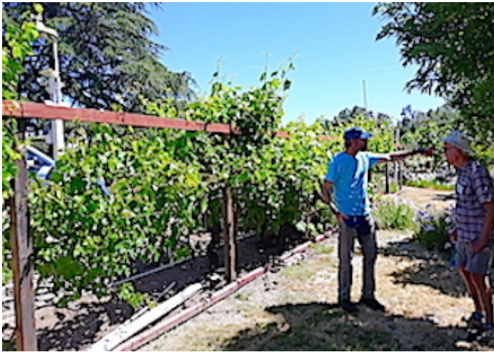
Matthew has finished the first stage of a support structure for the table grapes. In the future he will add a horizontal overhang to complete the grape arbor.
